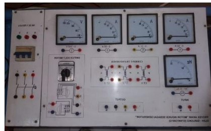
Gambar . Sumber Genset
