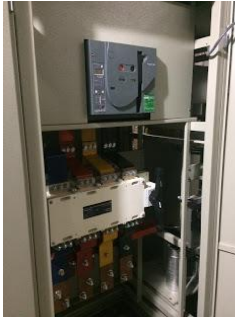
Gambar . Panel ATS AMF Motorized MCCB
