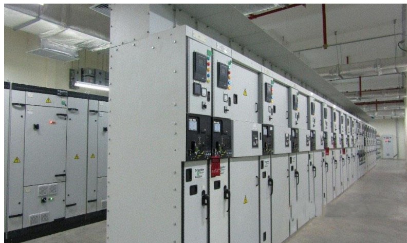
Gambar 16. MV SWGR 6.6 KV & MCC 4101 A/B
