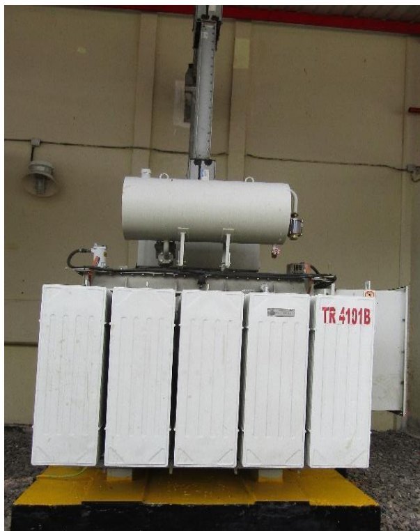
Gambar 11. Transformator TR-4101 B
