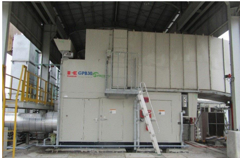
Gambar 7. Gas Turbin Generator
