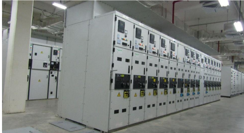
Gambar 15. Main SWGR 6.6 KV 4100 A/B
