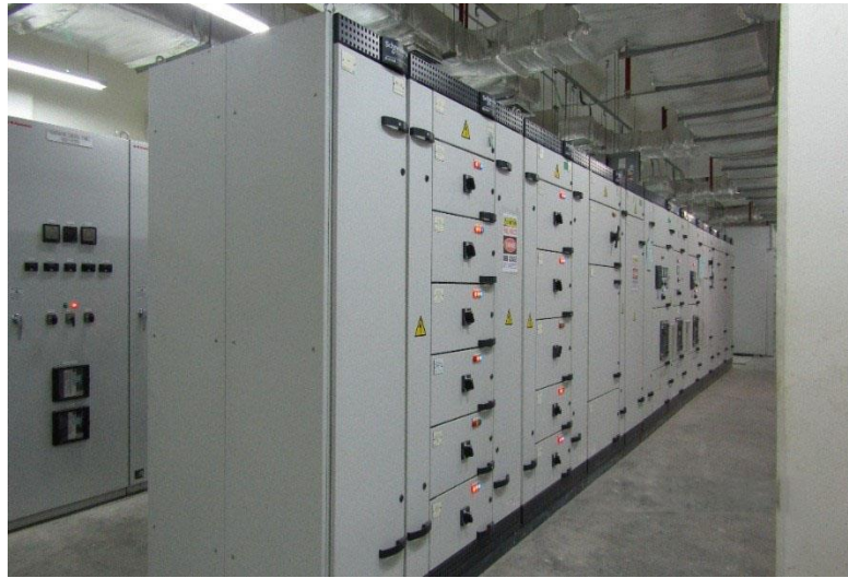
Gambar 19. Emergency SWGR 0.4 kV & MCC 4113 A
