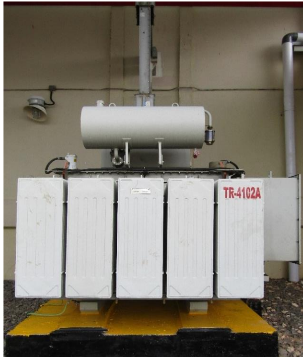
Gambar 12. Transformator TR 4102 A
