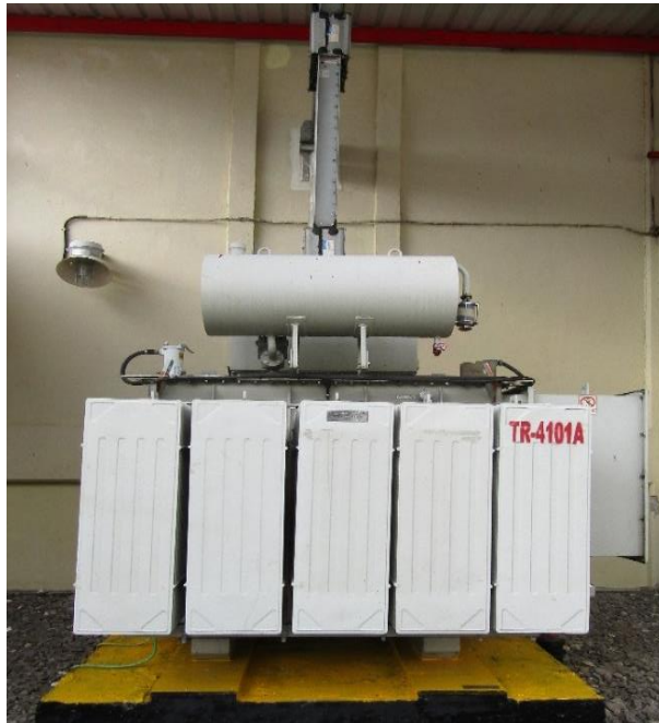
Gambar 10. Transformator TR 4101 A
