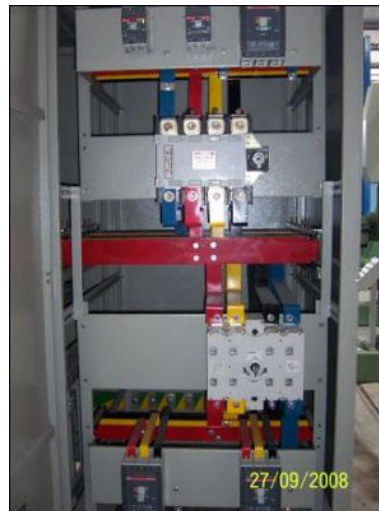
Gambar 8. Panel Change Over Switch
