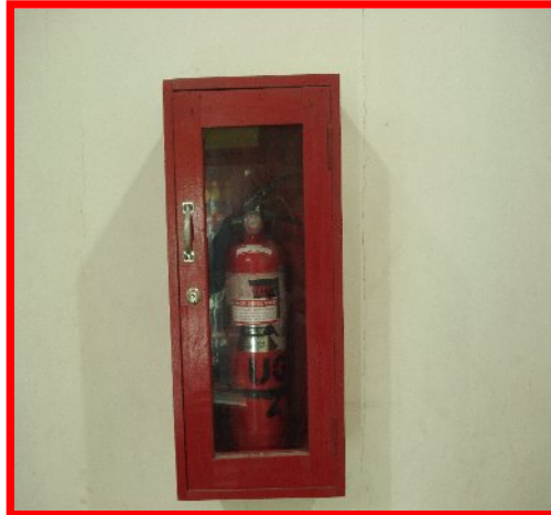
Gambar 16. Apar Dry Chemical
